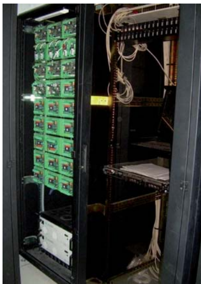
View of the access control bay
