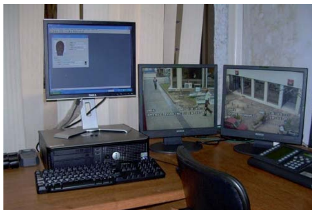
View of the surveillance and control post
