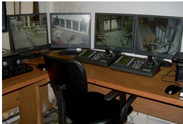
A view of the surveillance control post
