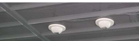
Over 100 cameras are connected to the access control system.
