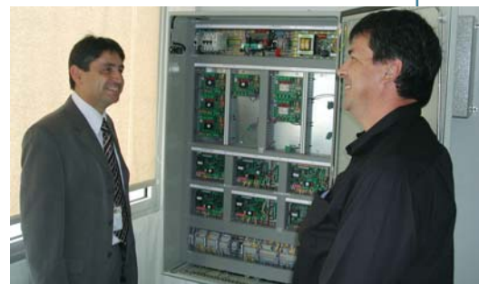
L. Bousquet (left), a technical executive at the airport, and Guy Patrick of Forclum, in front of the cabinet containing the intelligent controllers.
